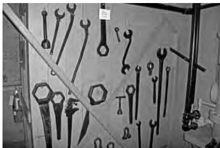
Boiler room maintenance tools.
