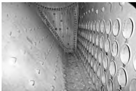
Steam boilers and inside the boiler.
